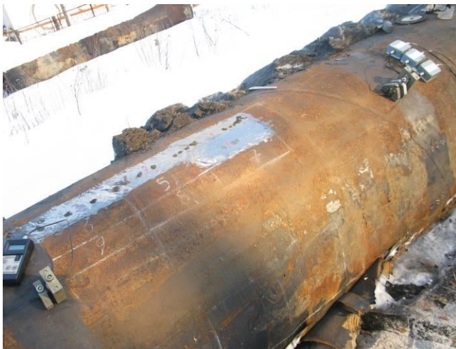
Fig. 6. A pipeline whose thickness was reduced up to 50% of its original value aside of the segment between the sensors.
