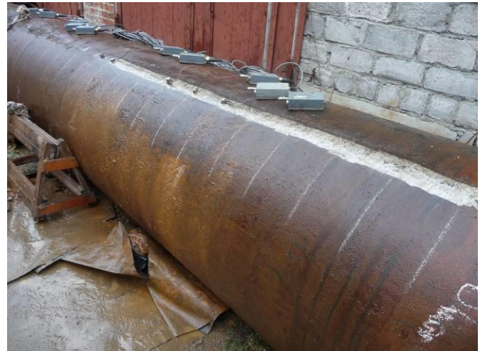
Fig. 7. A pipeline with the thickness profile in the form of the step-function.
